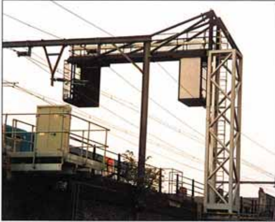
Cantilever Signal System
