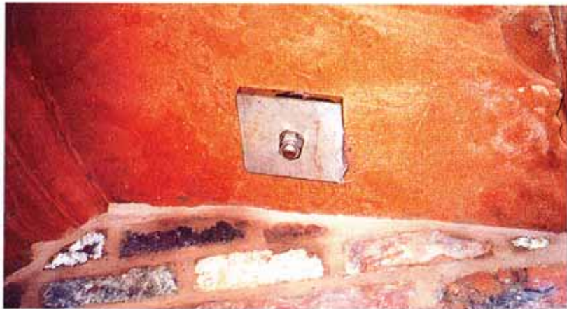
Roof bolt support to ballroom ceiling.
