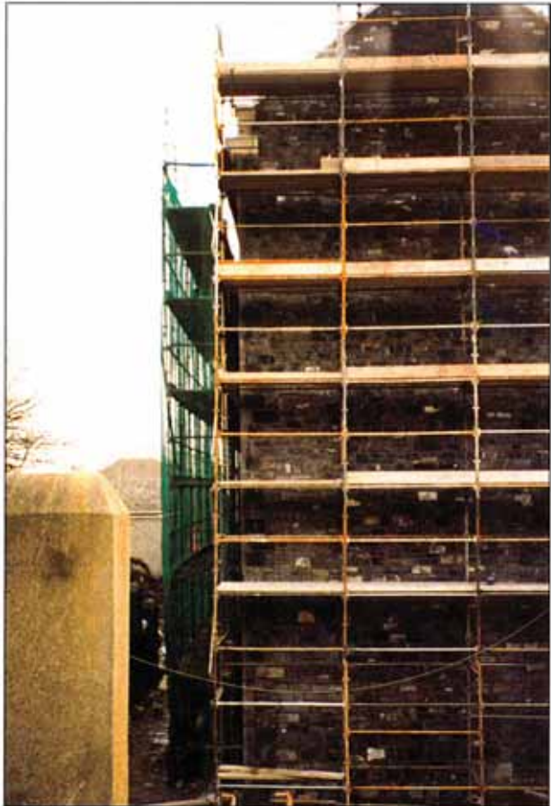
4 - 1800 x 30mm and 4 - 2200 x 30mm stainless steel anchors were used to stitch crack vertically up a five storey gable wall
