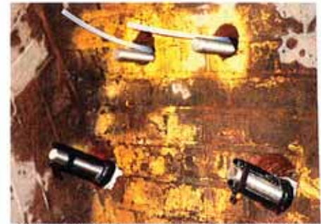
Shear anchors shown at the top and tension anchors at the bottom
