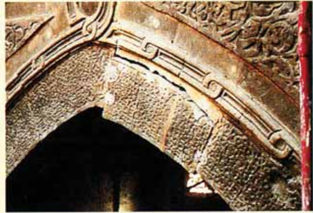
Seismic damage to decorative arches
