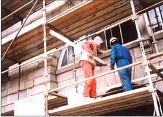
Anchor insertion approx 680 - 650mm x 10mm stainless steel anchors for facade retention
