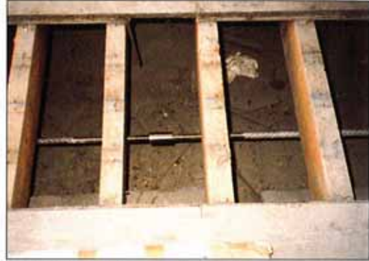
East block front and back arch tied with anchor assembly running from front arch to rear through floor
