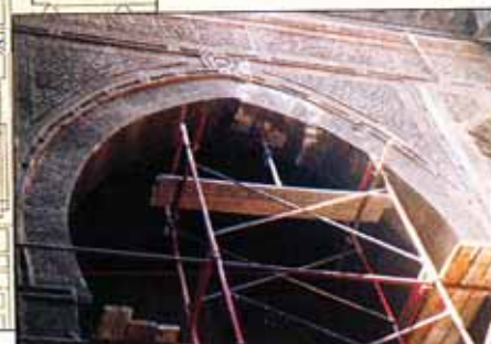
One of the four arches of the court being scaffolded prior to drilling and anchoring
